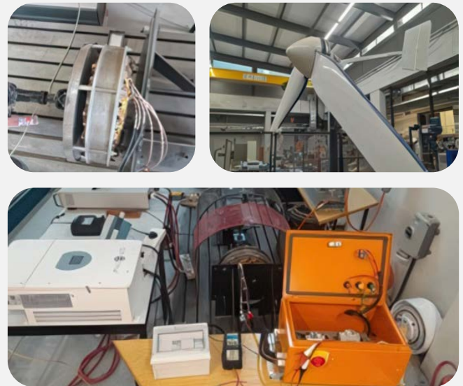
Photos of wind generator (left), wind turbine, nacelle and tail (middle), and lab tests showing the SUNSynk, generator and connection box (right). ^
