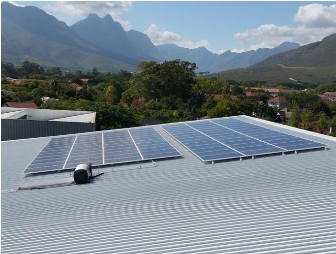
Figure 1: 22.5 kWp PV system at Stellenbosch University
