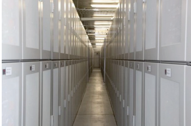
Inside the Tehachapi Energy Storage project.
