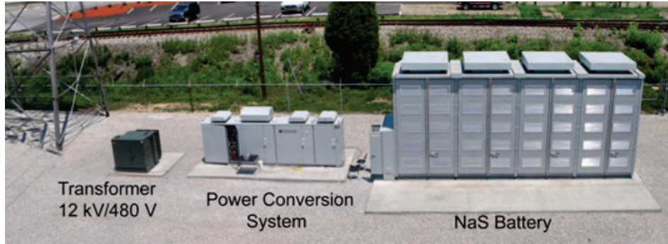
First S&C SMS Project \pm 1.25 MVA SMS on a 1-MW/7-hour NaS Battery
