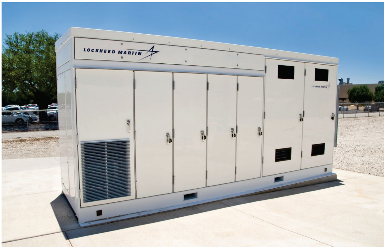
Lockheed Martin GridStar™ Li-ion 250-kW/540-kWh system in Grand Prairie, Texas.
