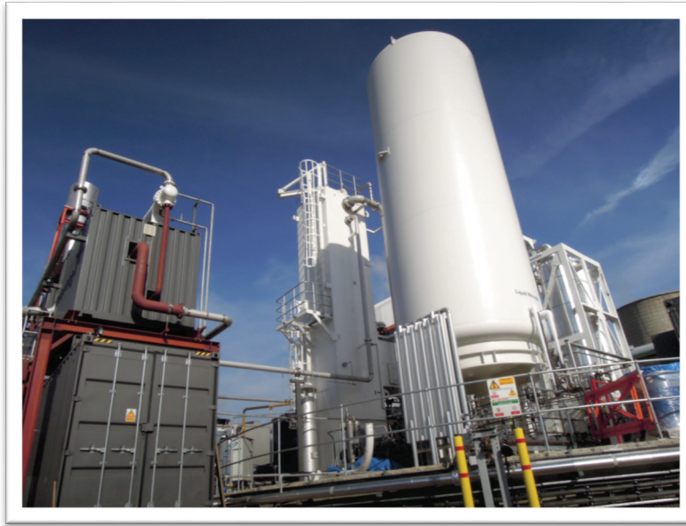
350-kW/2.5-MWh LAES Pilot Plant (courtesy Highview Power)
