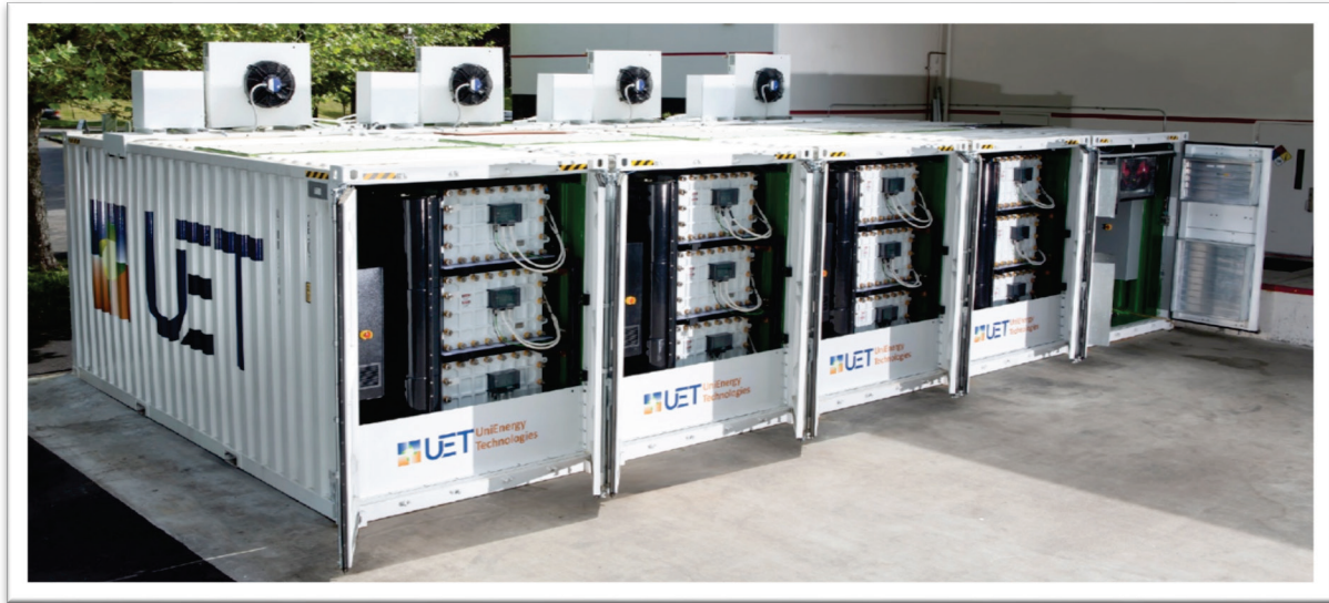
UET's Uni.System: 500 kWac and 4- to 12-hour discharge (up to 6 MWhac) (courtesy UET)
