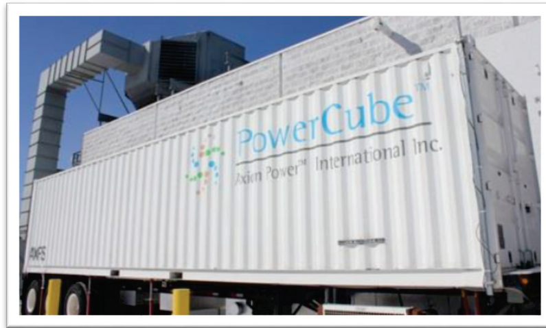
500-kW/360-kWh lead-carbon battery system in 40-foot container (courtesy Axion Power)
