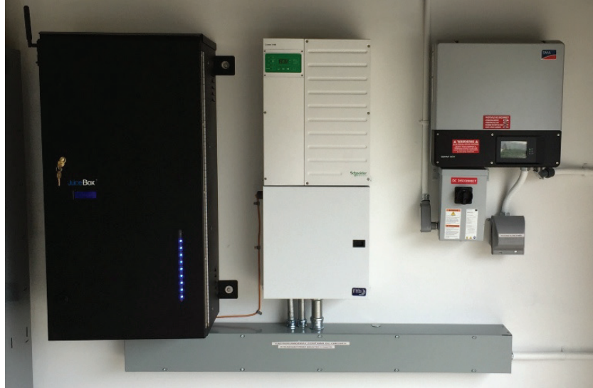
Adara Power's battery/controller cabinet (left) with inverter/wiring box (center) and solar controller (right).
