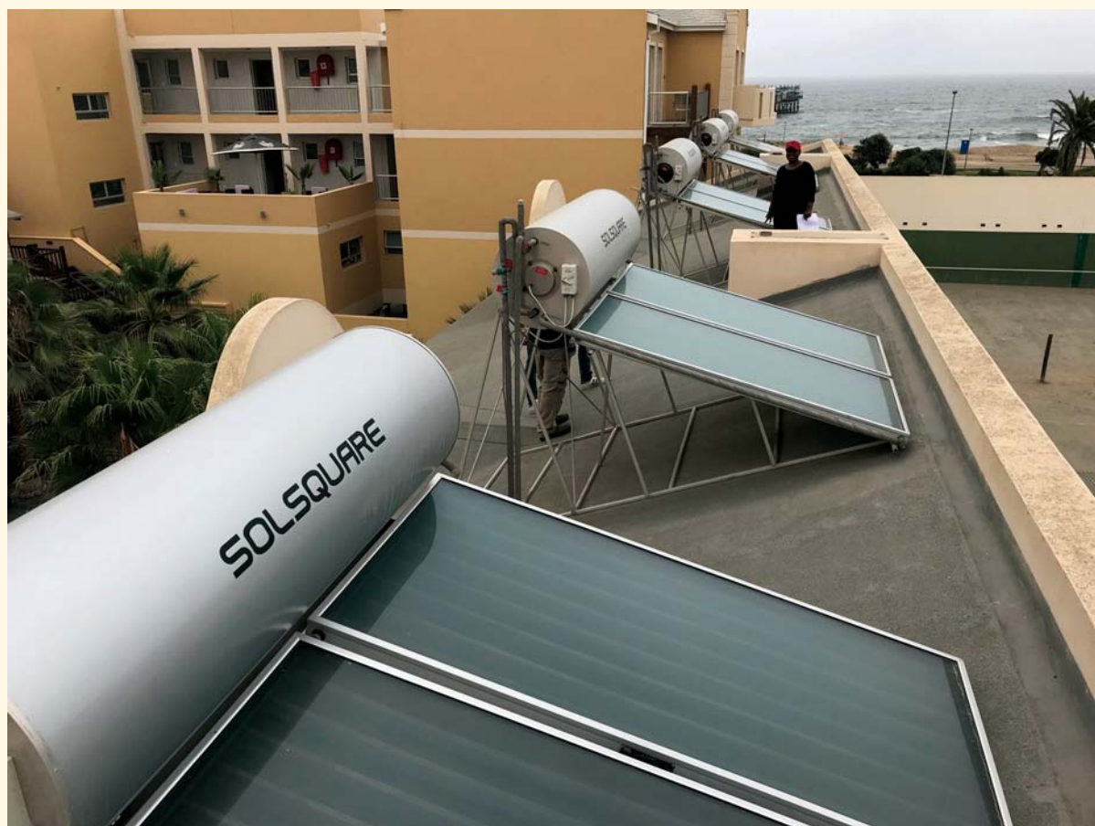
Thermosyphon systems at a hotel in Namibia.
