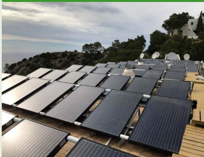
150 m 2 covered PVT collectors in Spain.
