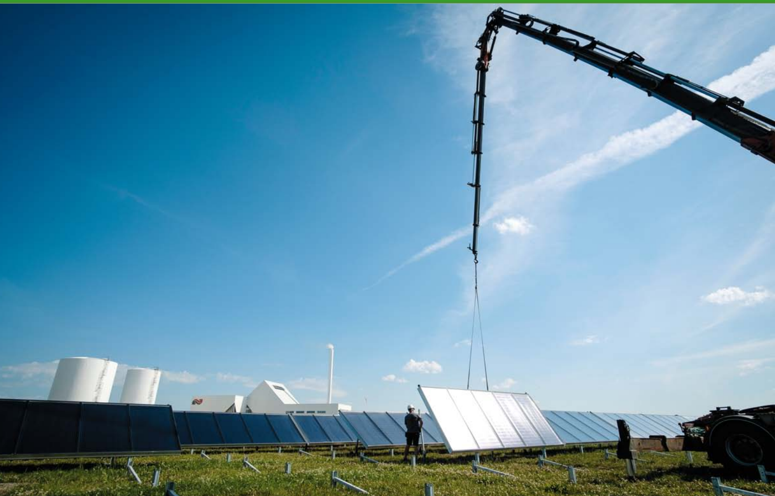
The Aabybro solar district heating system.
